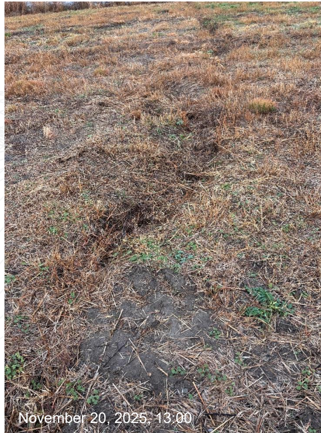
Erosion on the E side of impoundment cap. Photo taken facing west towards the impoundment cap. Approx. 4-6" deep.
