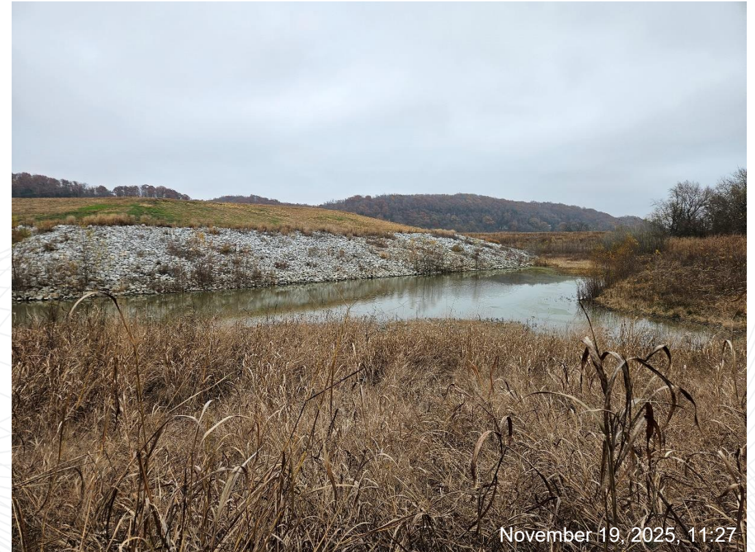
Ponded area in SW corner of site as viewed from APW-6D/S
