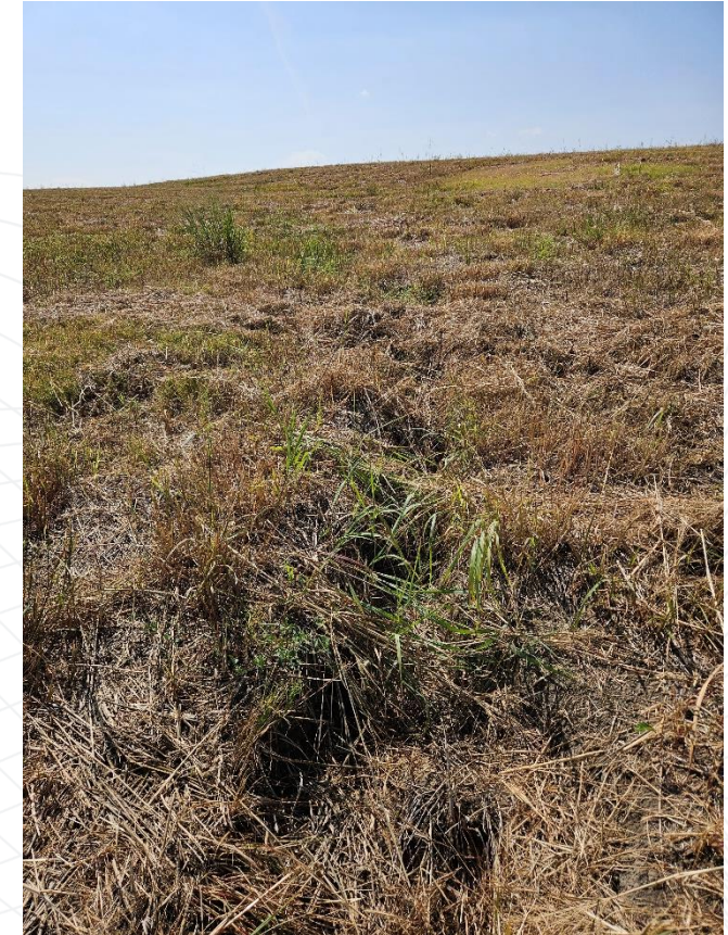
Erosion on the E side of impoundment cap. Photo taken facing west towards the impoundment cap. Approx. 6-8" deep.
