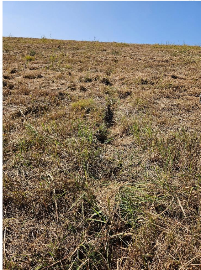
Erosion on the E side of impoundment cap. Photo taken facing west towards the impoundment cap. Approx. 4-6" deep.
