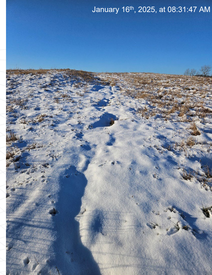
Erosion on the east side, roughly 4" deep, of impoundment cap. Photo taken facing west from the bottom of the impoundment cap.
