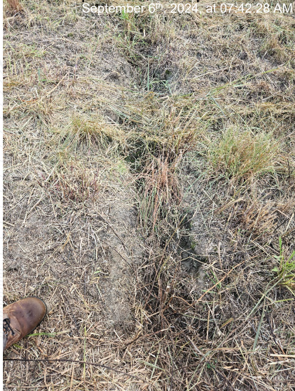
Erosion channel on north side of impoundment cap.
