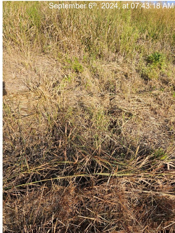
Erosion channel on west side of impoundment cap.
