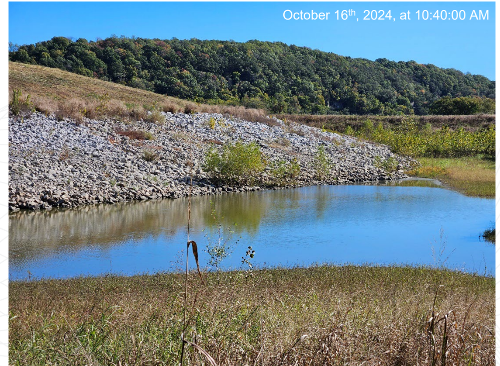
Ponded area in southwest corner of site as viewed from southwest corner.
