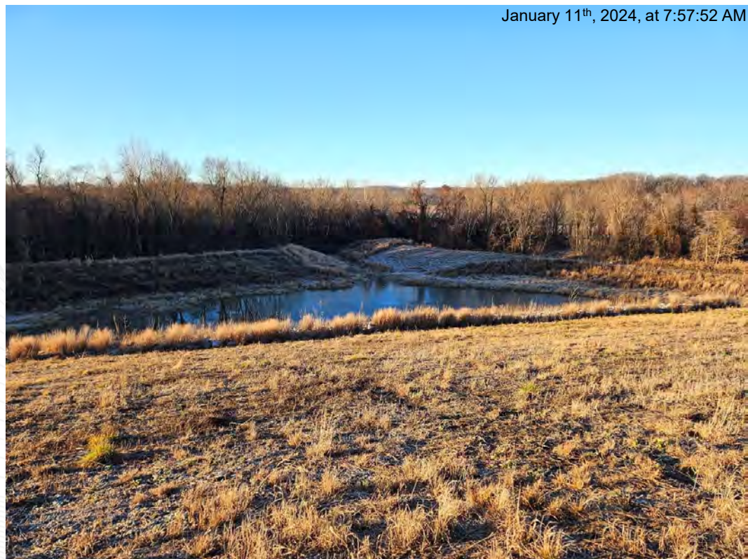
Ponded area in southwest corner of site as viewed from mowed impoundment cap.
