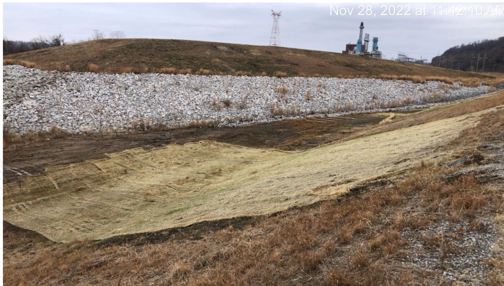
Facing north towards impoundment cap – repairs of fence and riprap undermining, and United States Army Corps of Engineers (USACE) levee section are visible.
