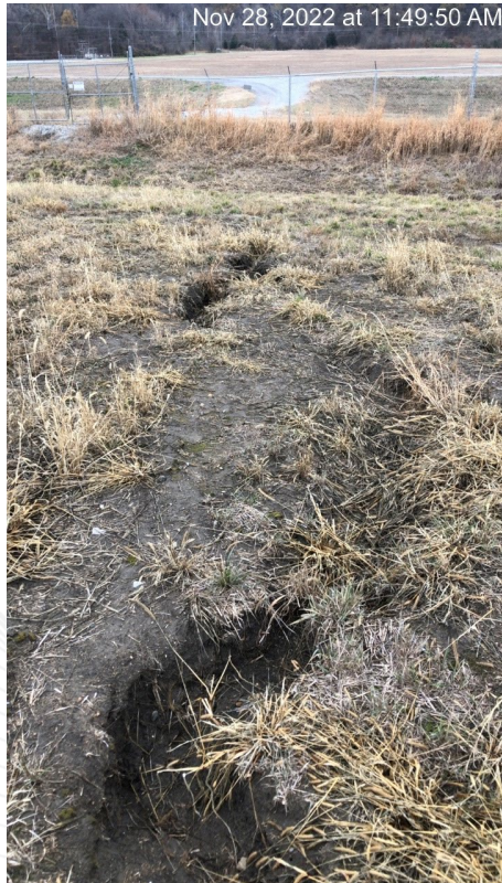
Erosional channel up to 9" deep. Facing east from center-east side of impoundment cap.
