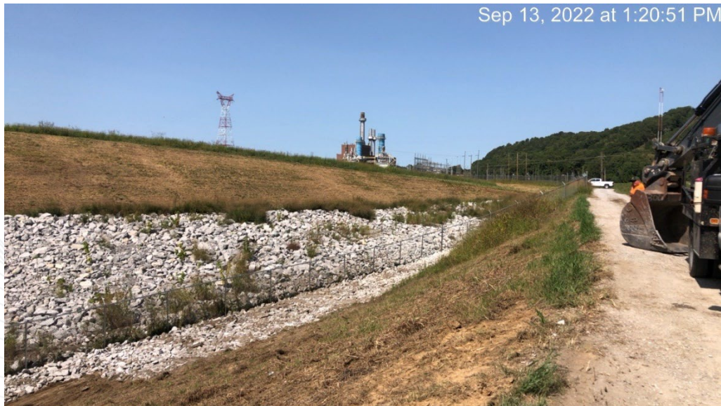
Facing north towards impoundment cap – repairs of fence undermining and riprap visible.
