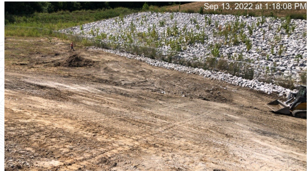
Facing southwest towards impoundment cap – repairs of fence undermining, levee, and riprap visible.
