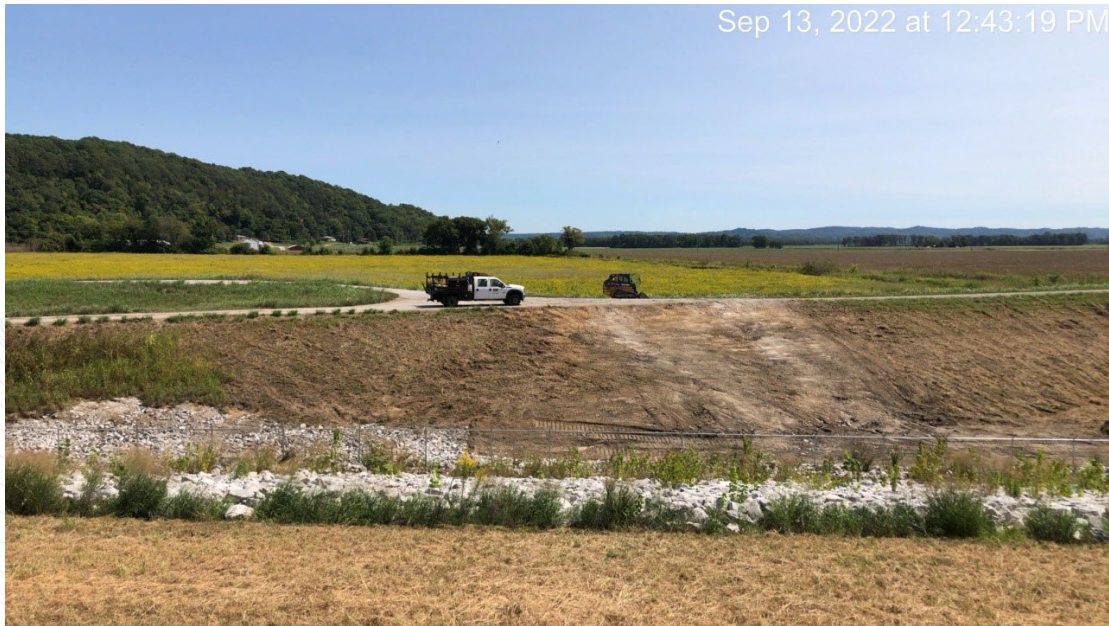
Repair of levee (both USACE and GTEC sections) underway as of 9/13/22 (facing east).
