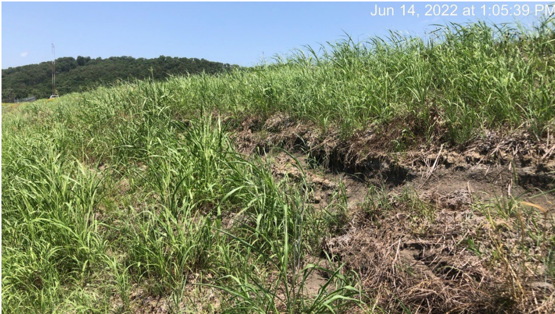
Close-up of slumped area.
