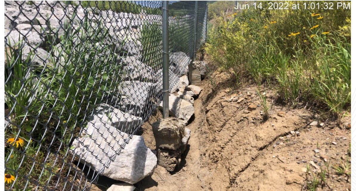
Undermined fenceline and riprap.
