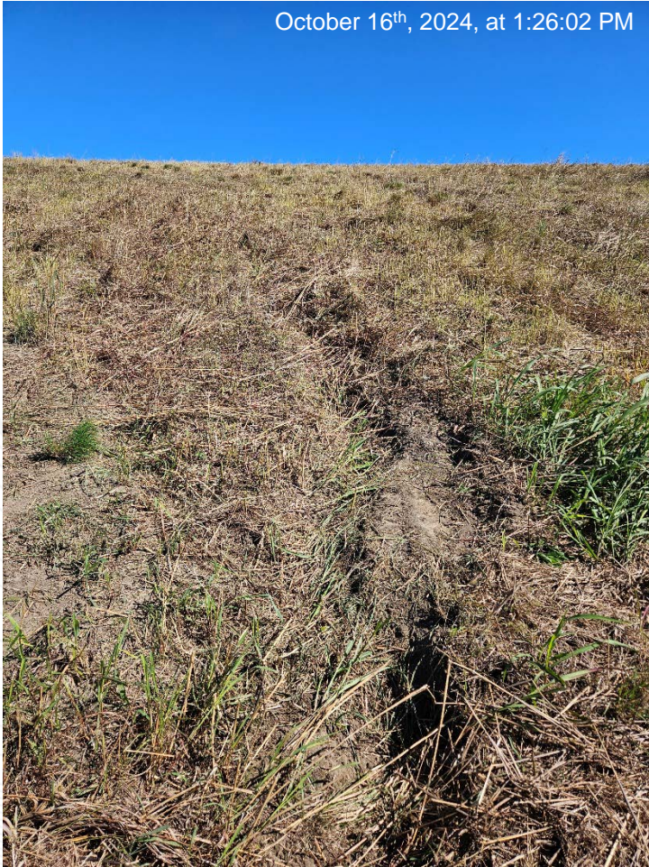
Erosion on the south side, roughly 6" deep, of impoundment cap. Photo taken facing north towards the impoundment cap.
