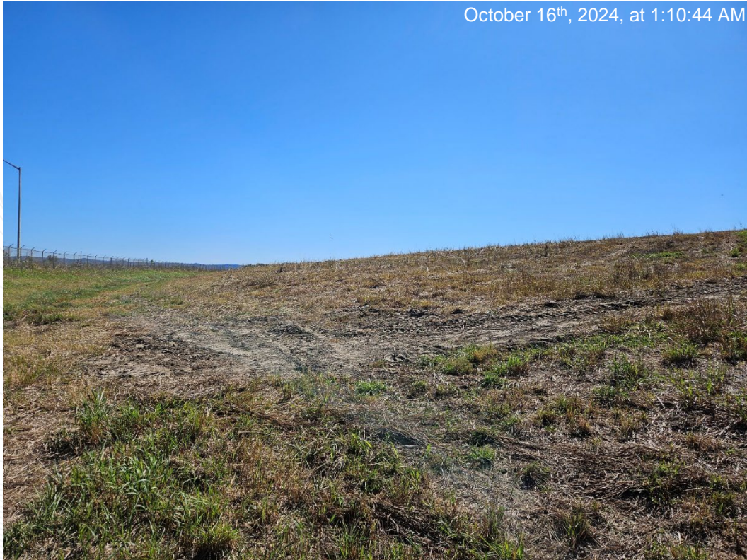
Erosion repairs made near the northeastern section of the impoundment cap. Photo taken from northeastern section of impoundment cap, facing south.
