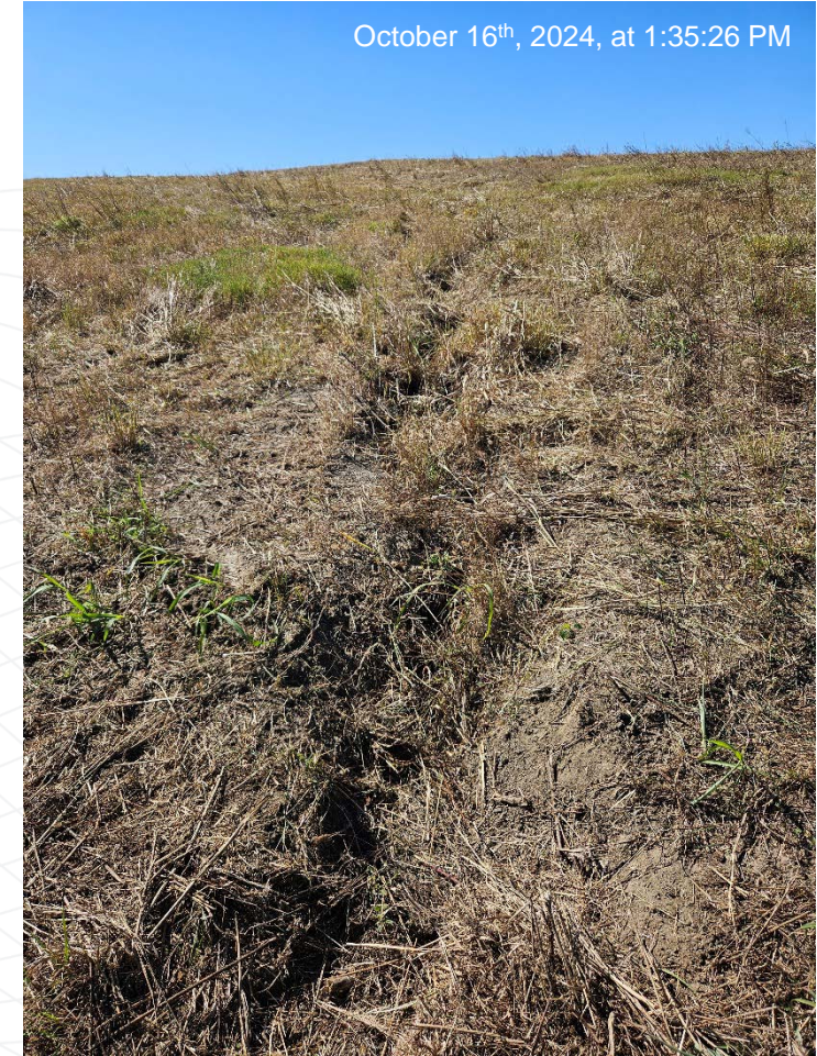
Erosion on the east side, roughly 4" deep, of impoundment cap. Photo taken facing west from the bottom of the impoundment cap.
