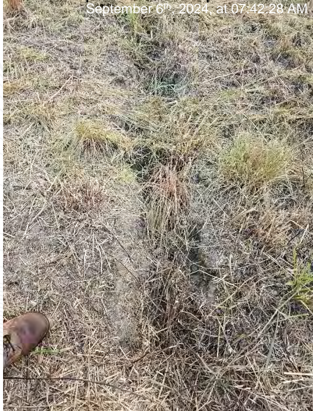
Erosion channel on north side of impoundment cap.
