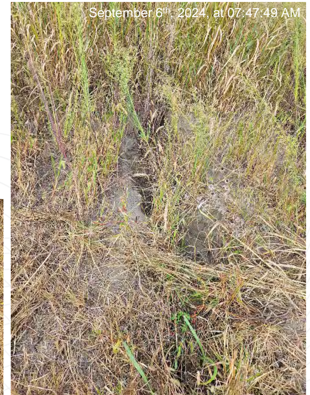
Erosion channel on east side of impoundment cap.
