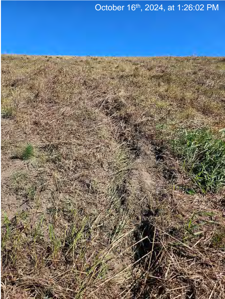
Erosion on the south side of impoundment cap. Photo taken facing north towards the impoundment cap.
