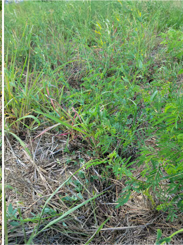
Erosion up to 9" deep - facing southwest from southern side of impoundment cap.
