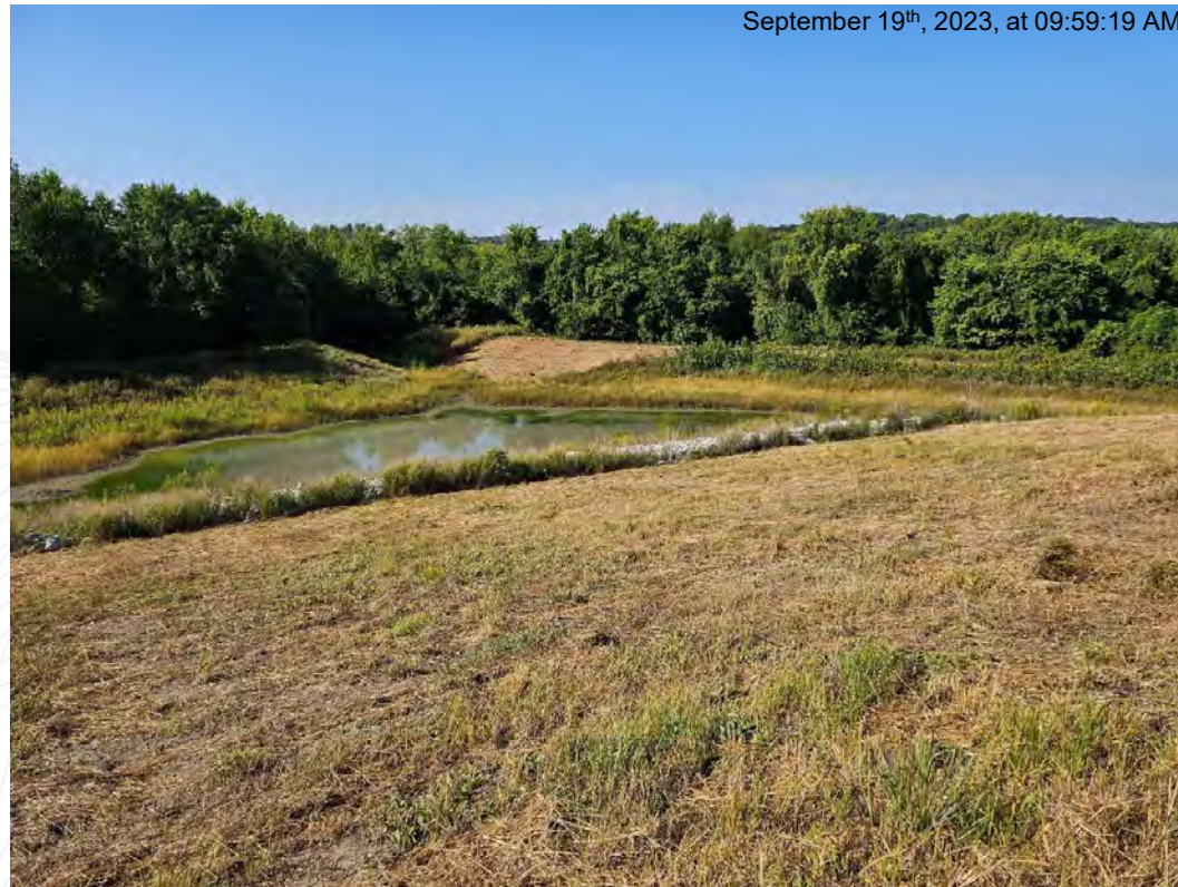
Ponded area in southwest corner of basin near the outfall, as viewed from mowed impoundment cap.
