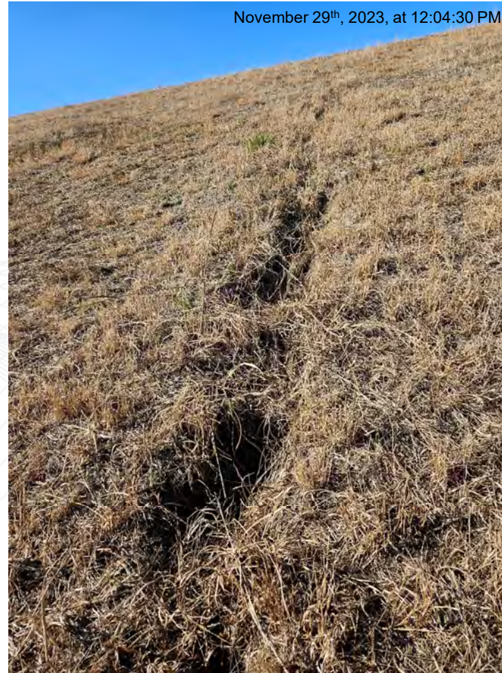
Erosion from western side of impoundment cap.
