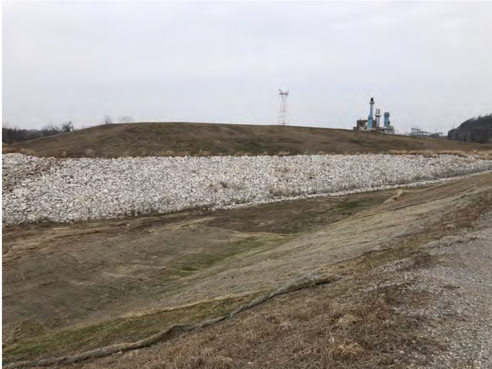
Facing north towards impoundment cap – repairs of fence and riprap undermining, and USACE levee section are visible.
