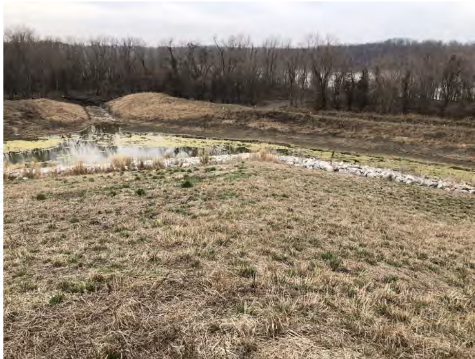
Ponded area in southwest corner of site as viewed from impoundment cap.
