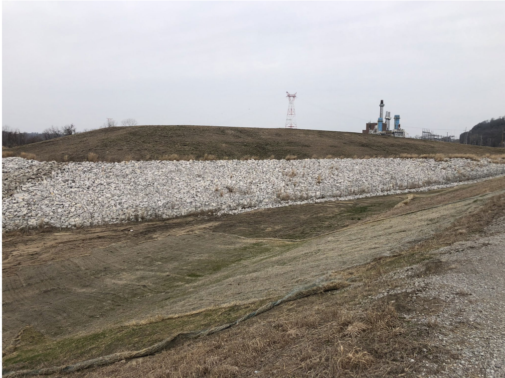
Facing north towards impoundment cap – repairs of fence and riprap undermining, and USACE levee section are visible.
