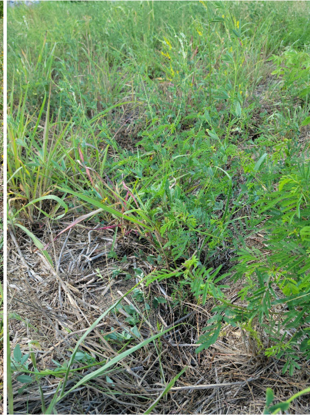
Erosion up to 9" deep - facing southwest from southern side of impoundment cap.
