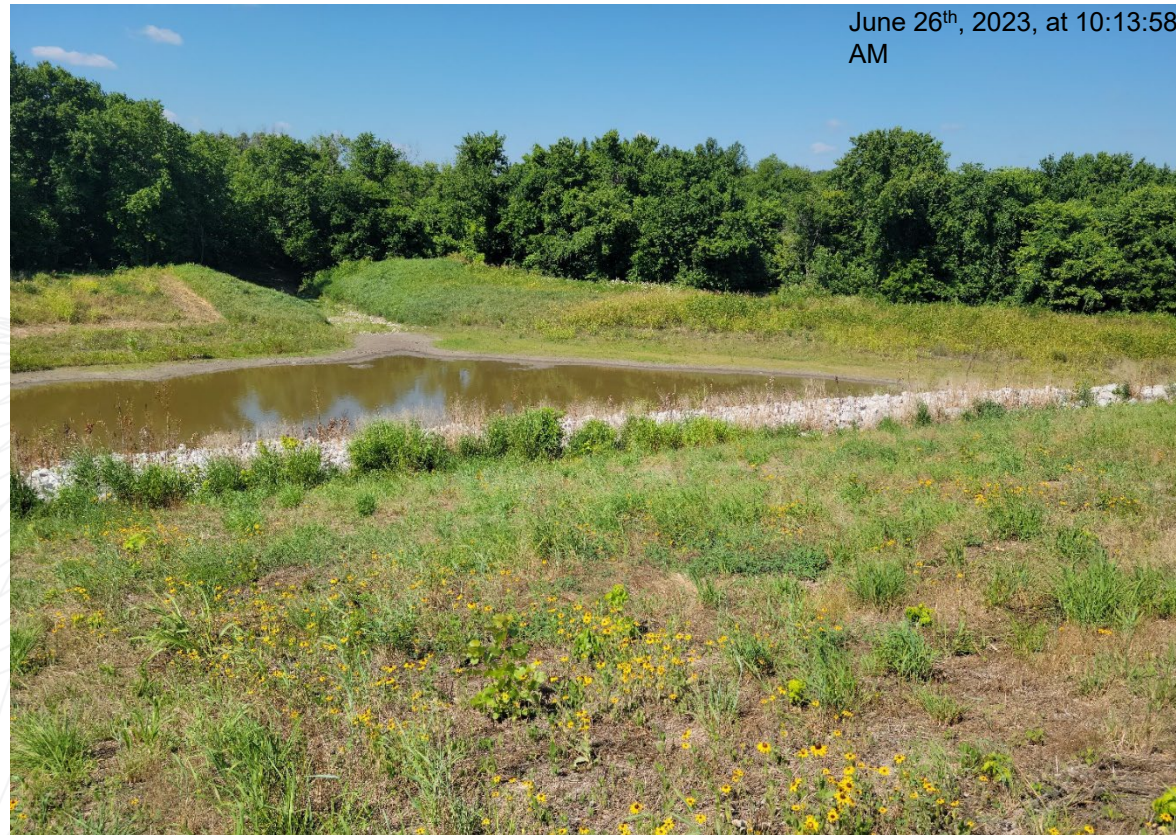
Ponded area in southwest corner of site as viewed from mowed impoundment cap.
