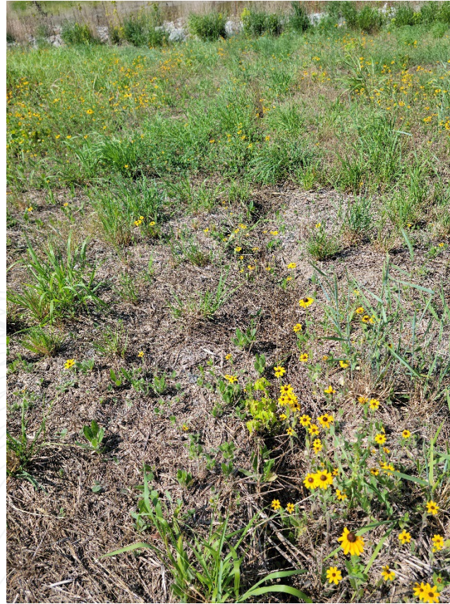
Erosion up to 9" deep - facing south from center-south side of impoundment cap.
