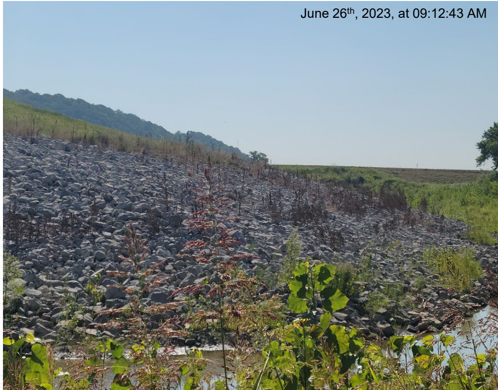
Facing east towards impoundment cap – dead/herbicide treated woody vegetation noted within riprap up to 1” diameter. Limited amount of live woody growth remains.
