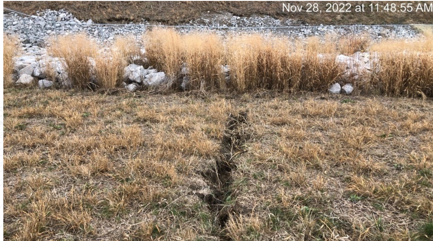
Erosional channel up to 9" deep. Facing east on southeast side of impoundment cap.
