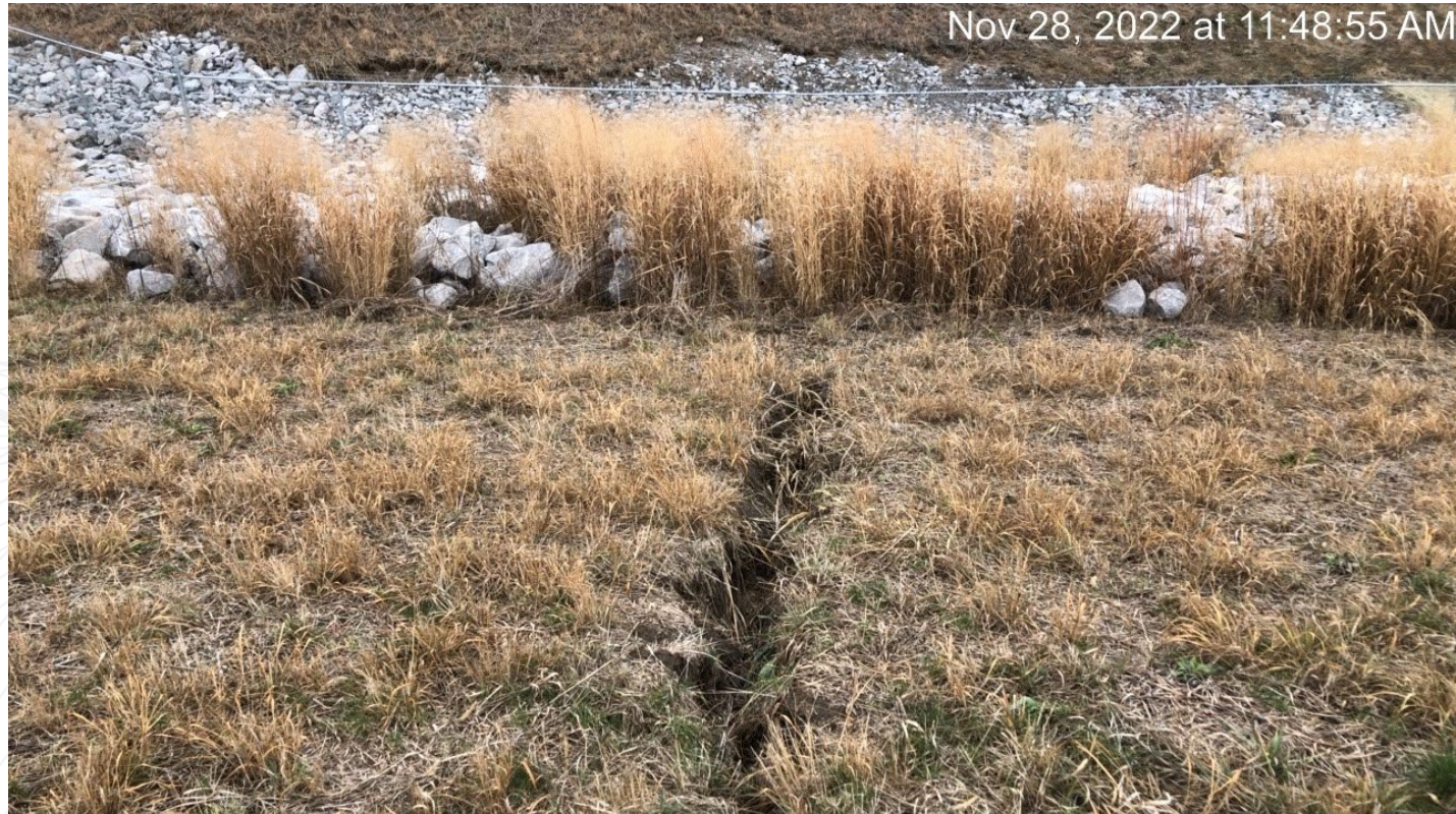
Erosional channel up to 9" deep. Facing east on southeast side of impoundment cap.
