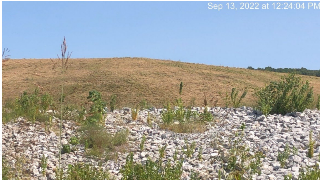
Southwest corner of the impoundment cap with limited woody growth (under 1" diameter) within riprap. Minor woody growth found within riprap along south, west, and northern sides of the impoundment.
