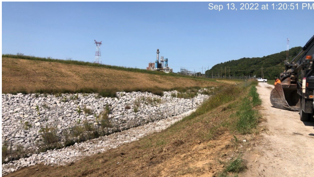
Facing north towards impoundment cap – repairs of fence undermining and riprap visible.
