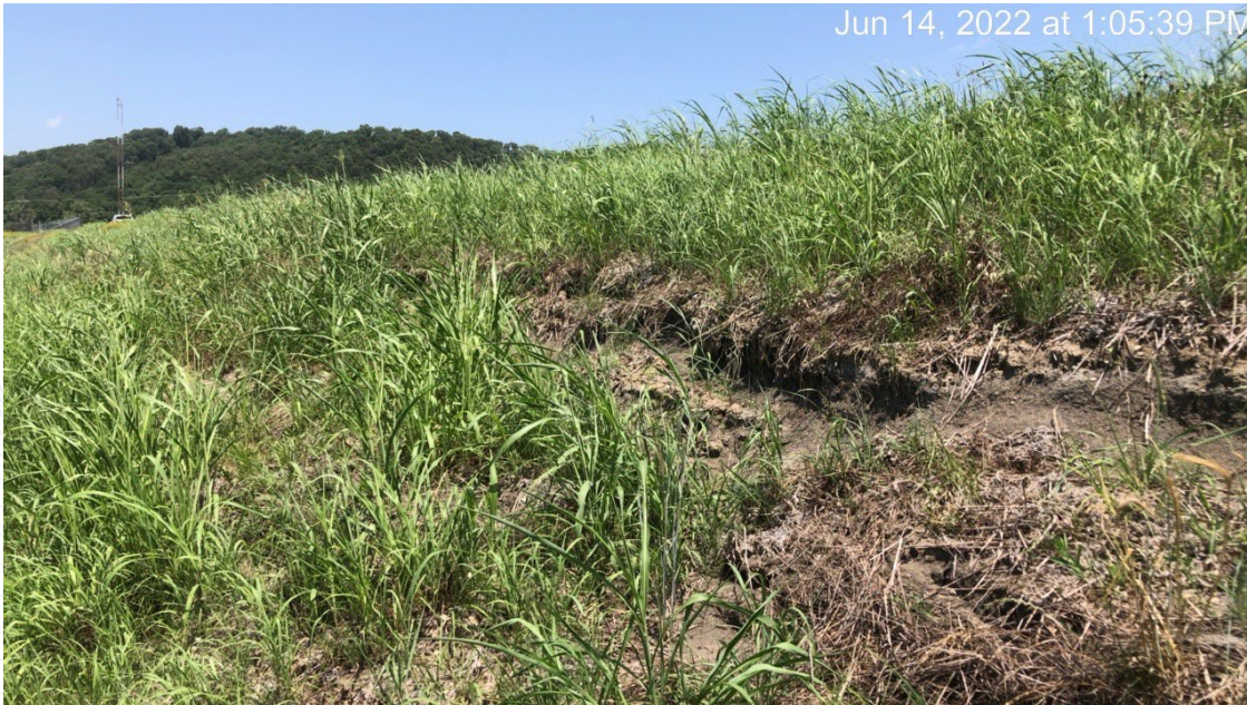
Close-up of slumped area.
