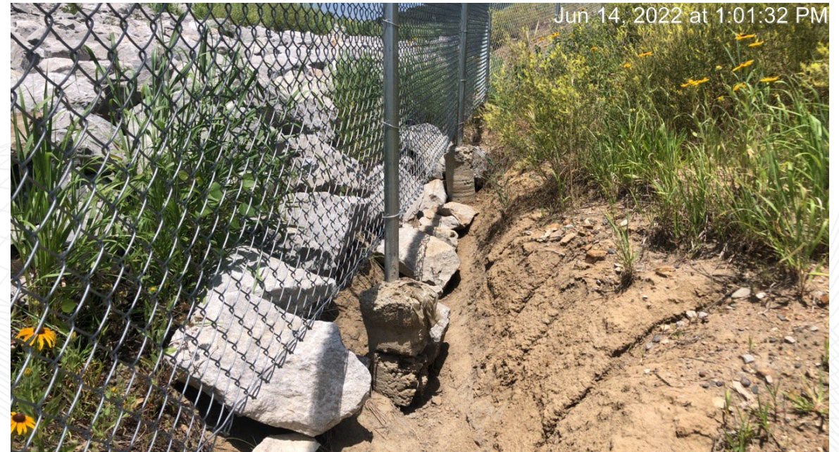
Undermined fenceline and riprap.
